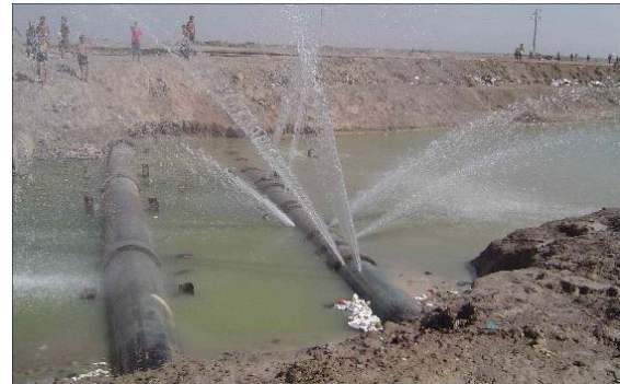
Leakage is not always so easy to detect
